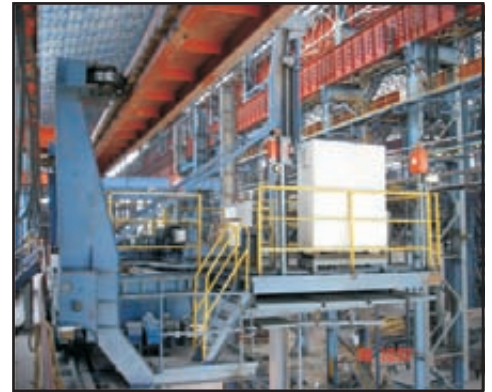
Mobile Nozzlex Addition System
